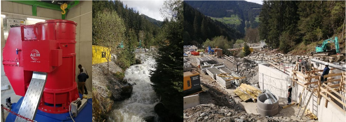
Figure 16: Site visit at Fotsch hydropower plant (on the left: hydropower generator, in the middle: hydropower water outlet, on the right: general view of the hydropower plant construction site)
